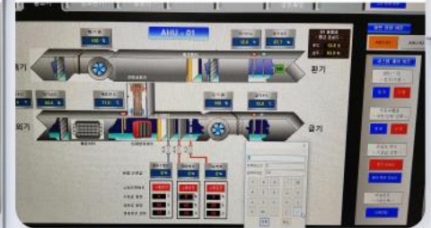
T.A.B (Testing Adjusting & Balancing)
